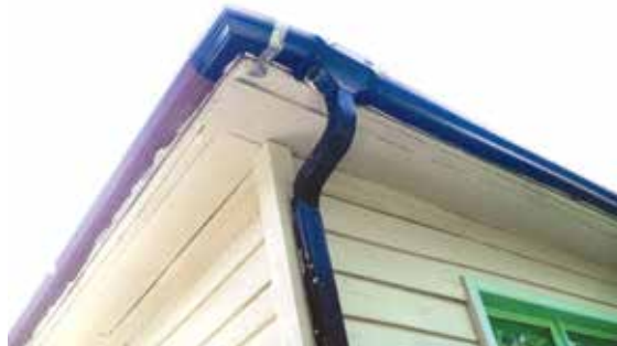
Poor repair of an eavestrough
