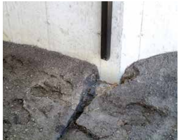
Downspout and grading problem.
