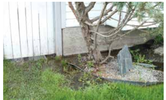
Water near a foundation.
