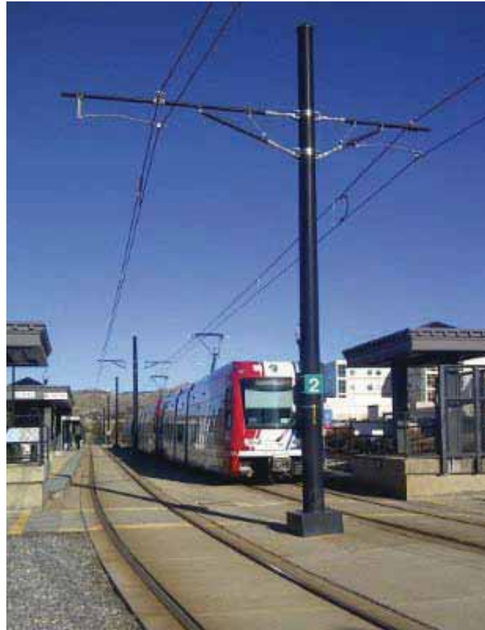
Examples of potential catenary poles
