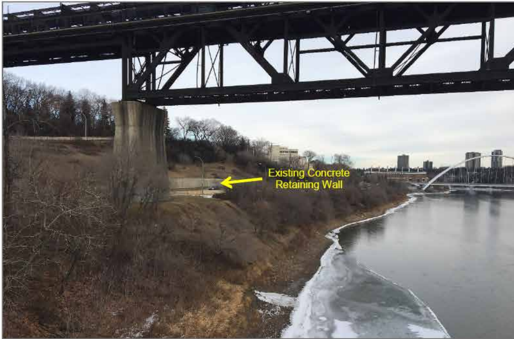
Photo 16: High Level Bridge Pier, Existing Concrete Retaining Wall and River Bank Slope
