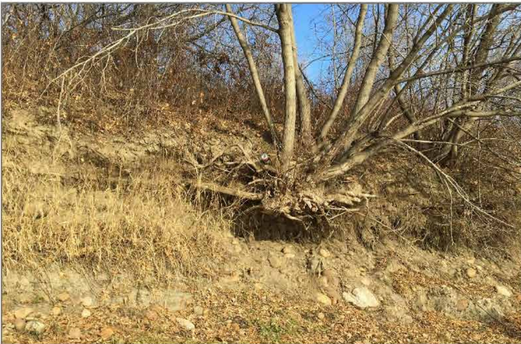
Photo 19: Eroded River Bank Slope and Exposed Tree Roots
