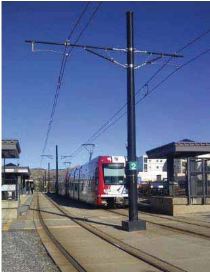
OCS provides power to the LRT vehicle. They are either located in the centre or on the side of the route. This location is determined by the space available and technical requirements.
