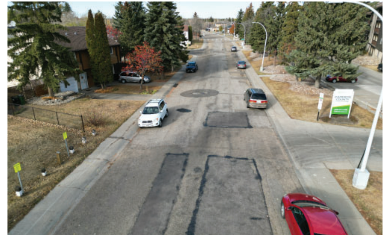
Local road with extensive repairs and patching.
