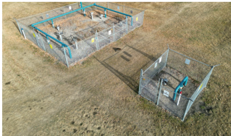
Pipeline access facilities near Hooke Road
