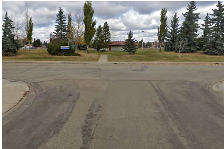
Sidewalk curb ramp aligned with centre of intersection, located on Lakewood Drive South
