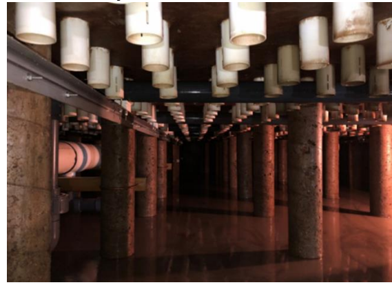
2. Filter Plenum Space
