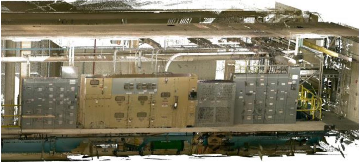
Filter Building Electrical Gear
