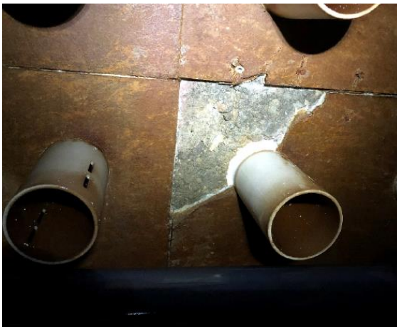
3. Spalled Piece of Transite Formwork
