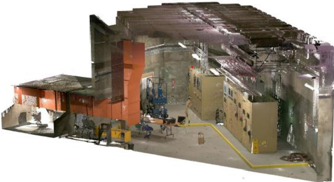
HLPB Electrical Gear
