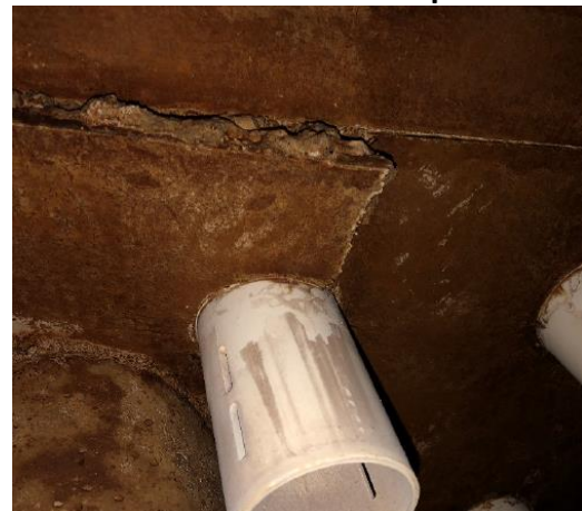
4. Separation of Transite Formwork
