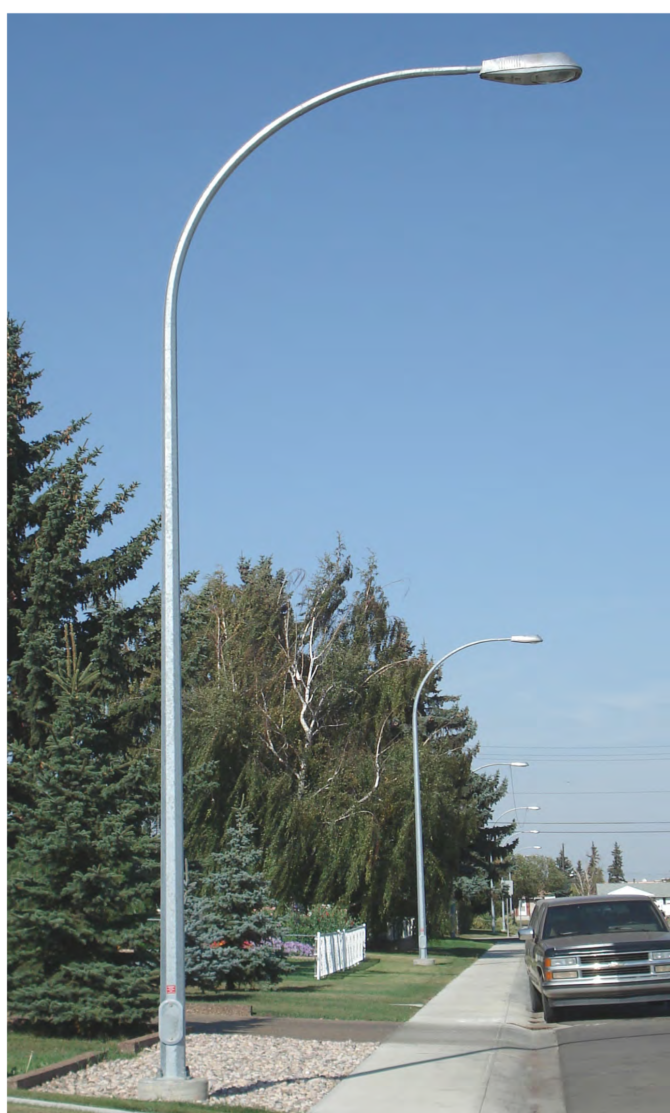
Galvanized street lights
