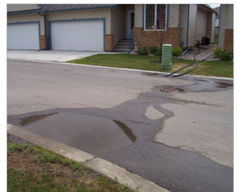
Settlement on private roadway near and around the catch basin at a multi-family property
