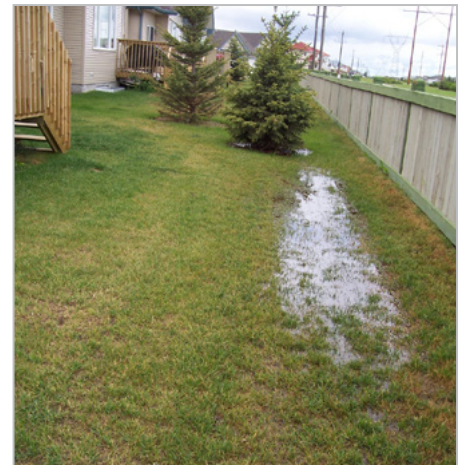
Ponding on an internal swale at a condominium property
