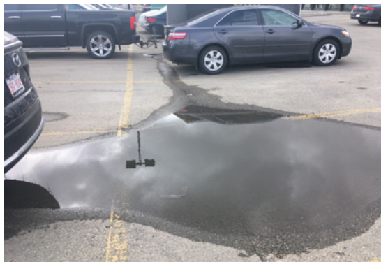
Settlement on parking lot on a commercial property
