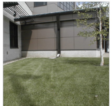
Downspout at a commercial building
