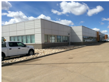
Grading away from a Commercial Building with Slab on Grade
