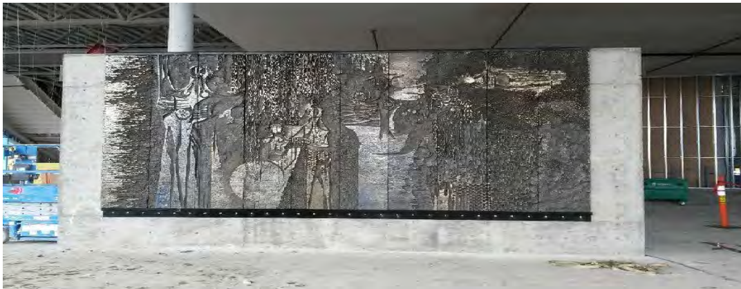
Untitled iron relief mural by Jordi Bonet, (1967) undergoing conservation treatment. All photos by David Turnbull Installation coordinated and executed by the EAC Conservation department at Millwoods Public Library
