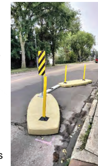
Adaptable curb extension on 102 Street and 82 Avenue, as part of the Ritchie Street Lab.
