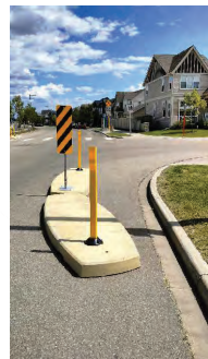
Photo of an adaptable curb extension on Allard Boulevard & Anthony Crescent, as part of the Allard Street Lab.
