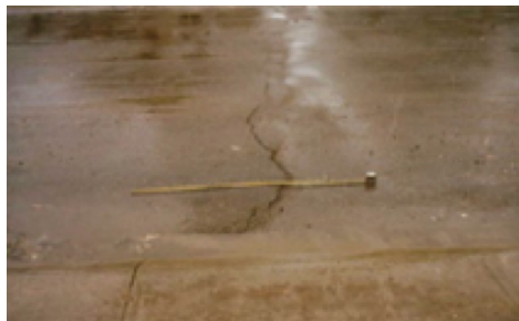
Open asphalt joints causing riding quality
