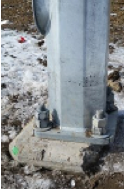
Damaged precast base
