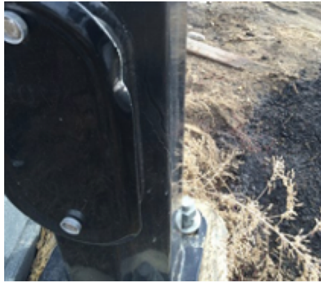
Damaged hand hole cover
