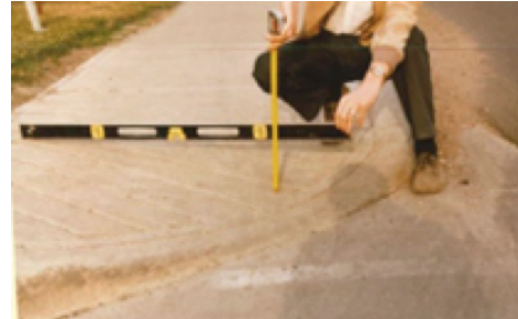
Curb ramp > 6.0% crossfall
