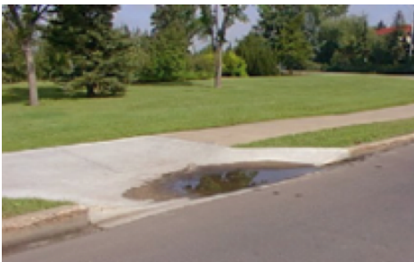
Standing water in crossing is unacceptable
