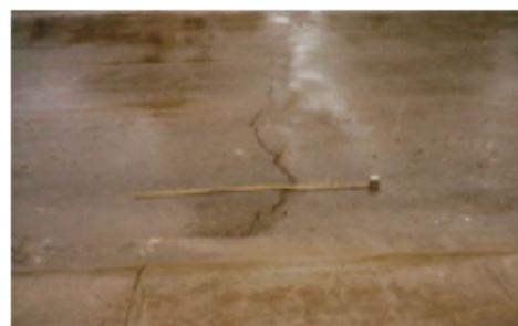
Open asphalt joints causing riding quality
