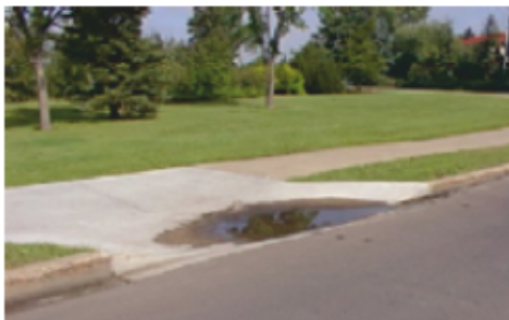
Standing water in crossing is unacceptable
