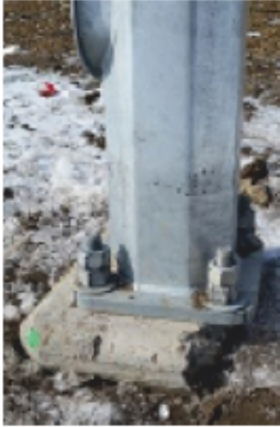
Damaged precast base
