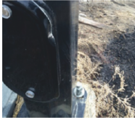
Damaged hand hole cover
