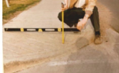
Curb ramp > 6.0% crossfall
