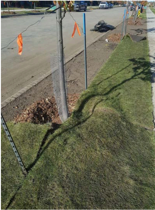
Construction Not Complete
