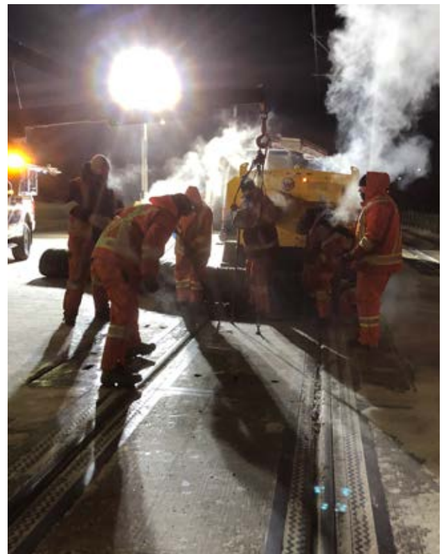
LRT track crew working overnight in -45^{\circ}\text{C} to repair a cracked rail
