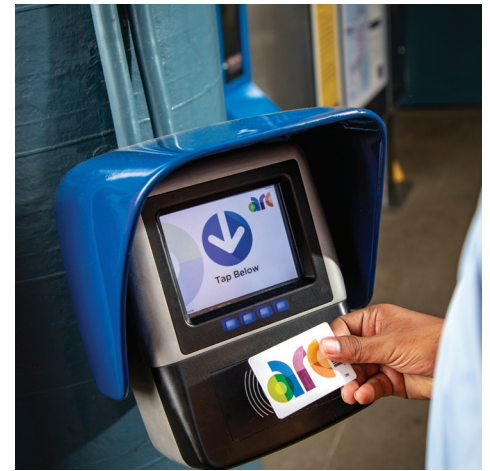
Arc fare validator at an LRT station
